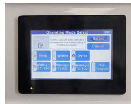
Automatic SO2 Dosing System
